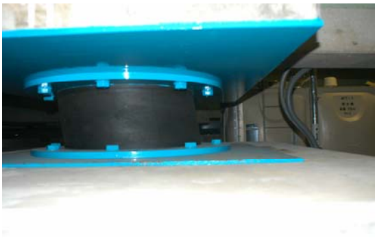
Photograph 2.1 Deformed elastomeric isolator.
