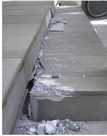
Photograph 3.2 Damage around the entrance.
